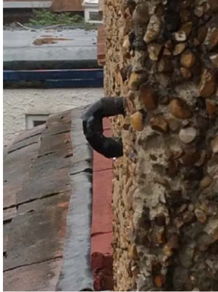
Water discharging at PRV terminal
