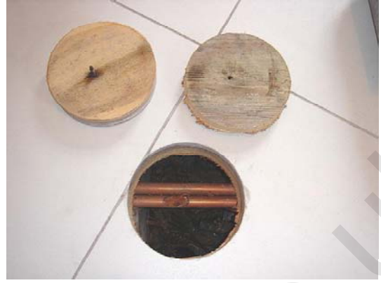
Nail punctured leaking
