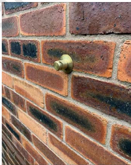
No water discharging at PRV terminal
