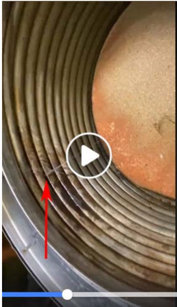
A pin hole at a main heat exchanger
