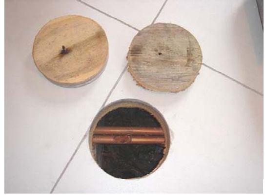
Nail punctured leaking
